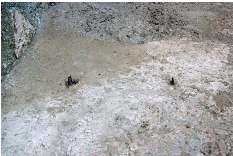
Fig. 20. Pompeii VI 14, 21-22, shop 21: pieces of iron fixed in the floor; remains of unidentifiable work installation.
